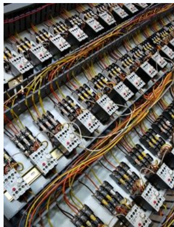
Motor control gear, wired and terminated
