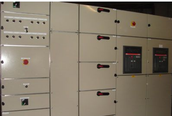
Main switchgear and distribution boards
